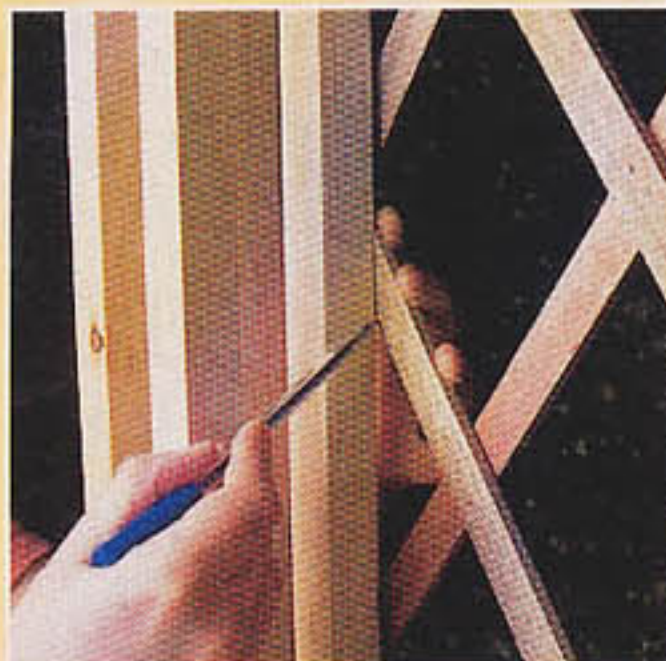
18 Hold the trellis against the outer face of the columns, then mark and trim it so that it slips into place between the timbers
