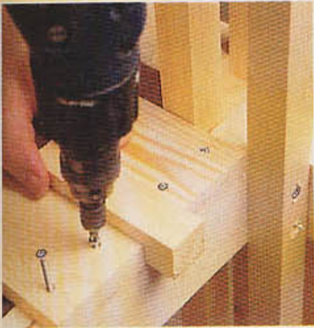
13 Use a piece of timber as a spacer between the seat slats. Take care not to split the ends as you screw them
